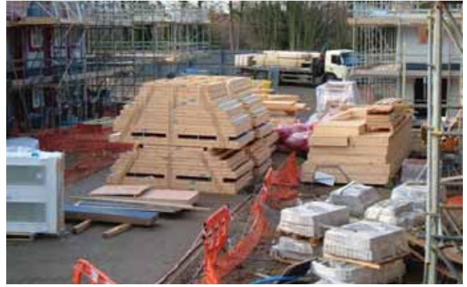
The use of timber frame in a development creates a number of advantages
