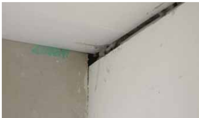
Detailing, finishing and sealing between the walls, floors and ceilings that make up the air barrier is critical to achieving air tightness
