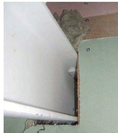
More services mean more penetrations through the air barrier and therefore more opportunities for air leakage
