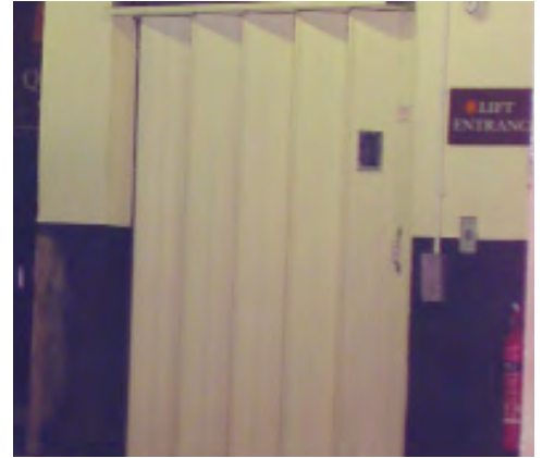
The goods lift at the centre of the case
