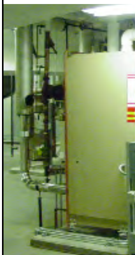
The EU Directive on Energy Performance of Buildings calls for the regular inspection of boilers
